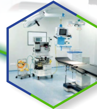
Central Oxygen and Suction Facility
